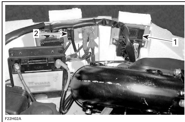
1. VCM 2. Main fuse
